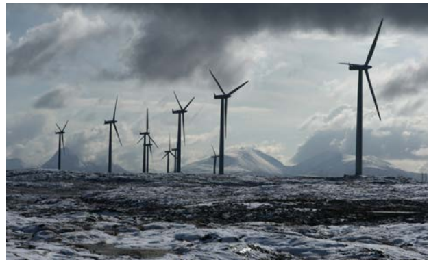
Smøla Wind Farm. Photo: Statkraft / flickr
